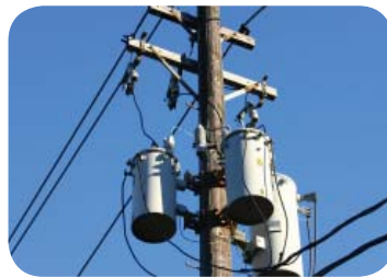
Utility equipment management.
