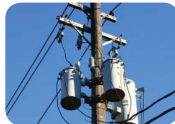
Utility equipment management.
